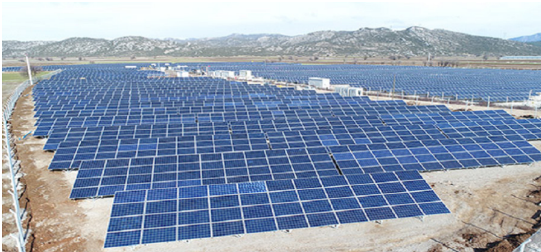
Figure 4: Installed 5 Mwh Solar Power Plant with Photovoltaic Cells in Antalya-Türkiye
