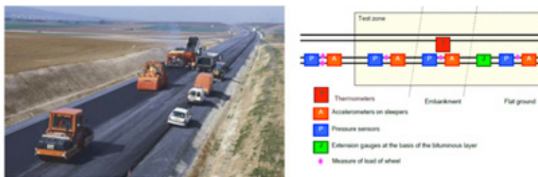
Figure 6. Laying of the asphalt layer of the SNCF test section and instrument layout plan in the test area (Wikizero 2019)
