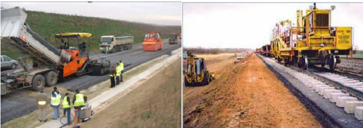
Figure 5. Paving of asphalt pavement layer on Italian high-speed railway line (Rose et al. 2015)
